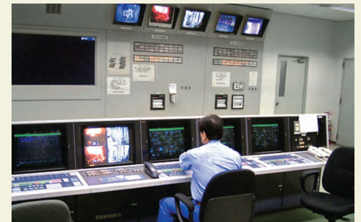
●中央制御室 工場全体の状態を常に監視し、集中操作します。 The entire plant is monitored and controlled from a central control room.
